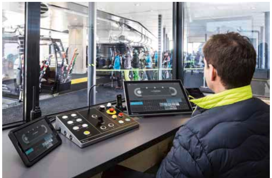
This way, the operator has an overview of both the cable-car status and the passengers at the same time.
