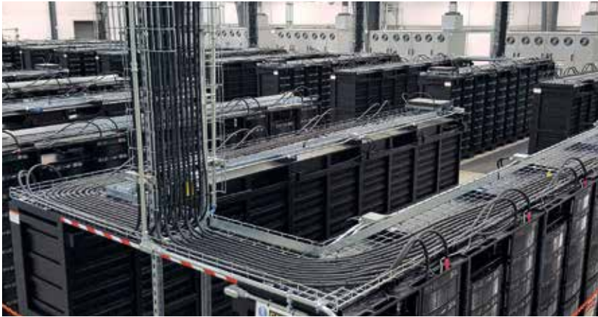
▲ A look inside the Notrees 36 MW battery park – the largest battery storage system in the USA connected to a wind farm.
