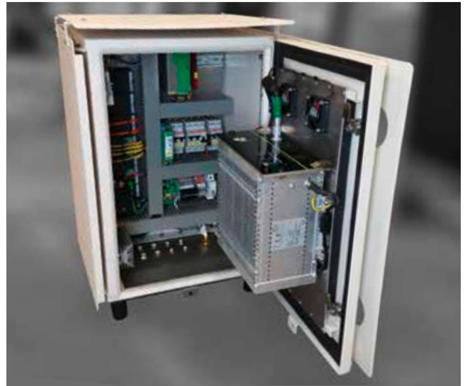
▲ The M1 controller is installed in the control cabinet.
