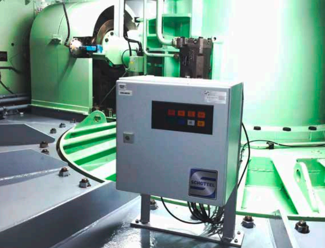
◀ In the engine room the sensors are more easily accessible for maintenance purposes.
