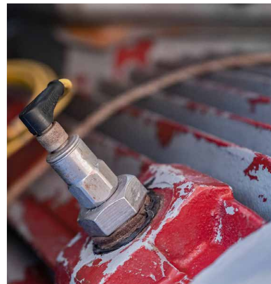
▼ Bachmann BAM100 sensor mounted on the electric motor
