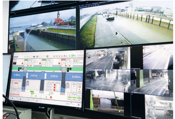
The Cuxhaven sea lock control room: Several operators can work simultaneously thanks to atvise® web technology.
