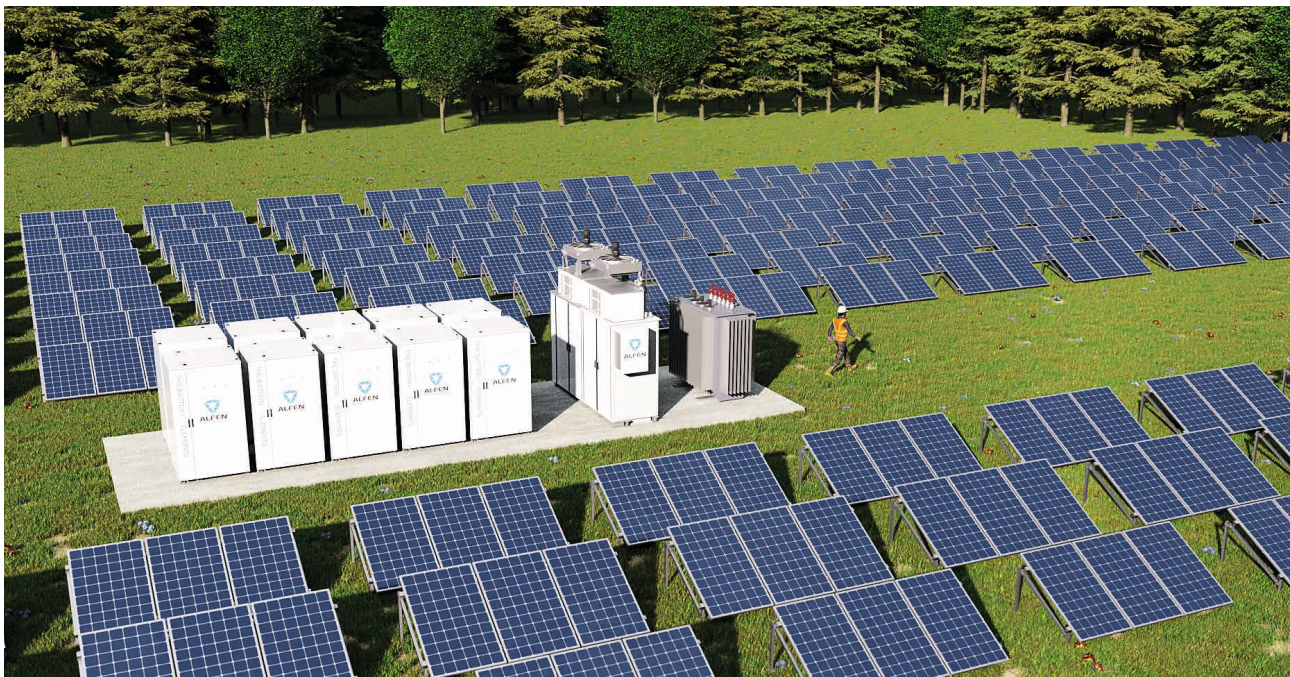
For industrial applications with power greater than 1 MW, Alfen offers the modular expandable solution TheBattery Elements as an End-2-End solution, including local grid embedding and network integration.
