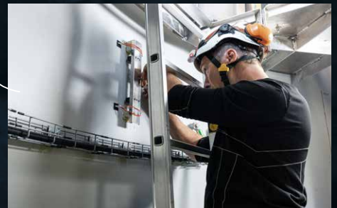
Completely relaxed, despite being 100 meters above "ground": Thomas Stauche from Bachmann's offshore team mounts a Cantilever Sensor inside the wind turbine tower.
