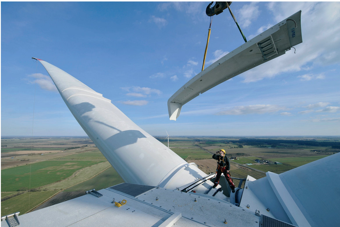
▲ One of the most powerful wind power systems in the world: 6M series from REpower Systems.
