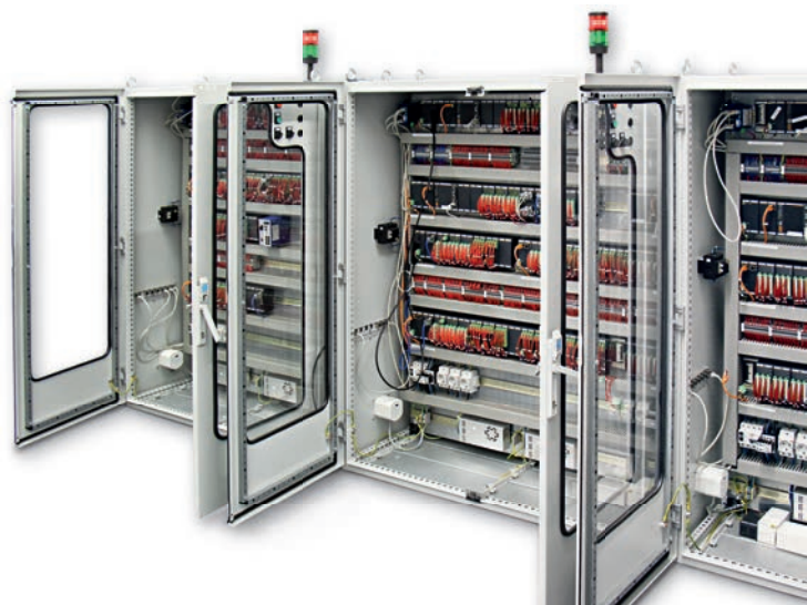
► Joint tests: The controller configurations for Senvion have been set up in the Bochum technical office of Bachmann electronic.
