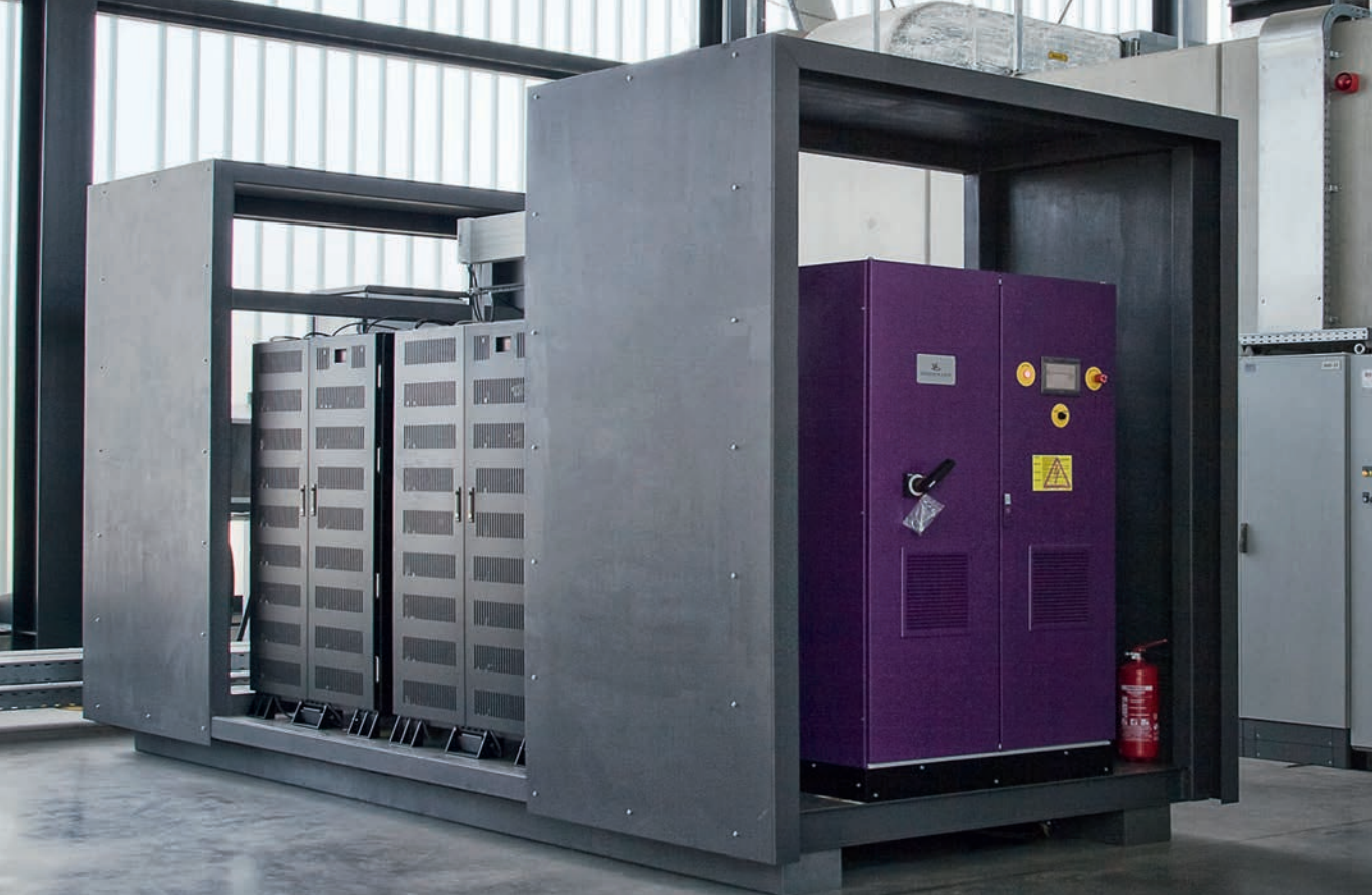
▲ Modules above head height: Battery storage systems based on lithium-ion technology, as used in the WEMAG battery park in Schwerin.
