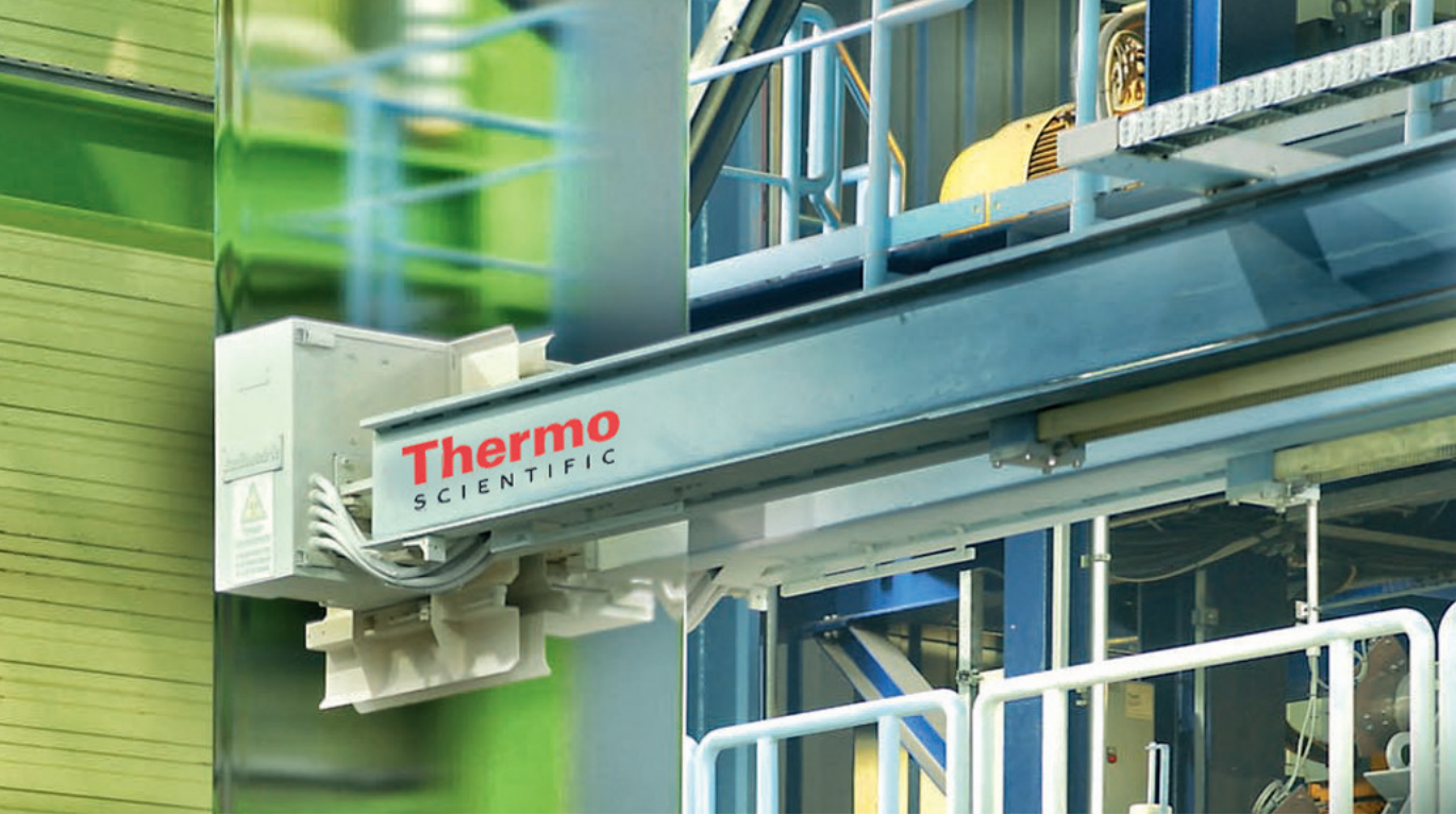
▲ Thermo Scientific RM310EH X-ray fluorescence hot coating weight gauge installed directly over the zinc pot of a hot dip galvanizing line. The system contactlessly measures the surface weight of the zinc coating applied in liquid form to the steel strip. The zinc coating is regulated according to the measured value.
