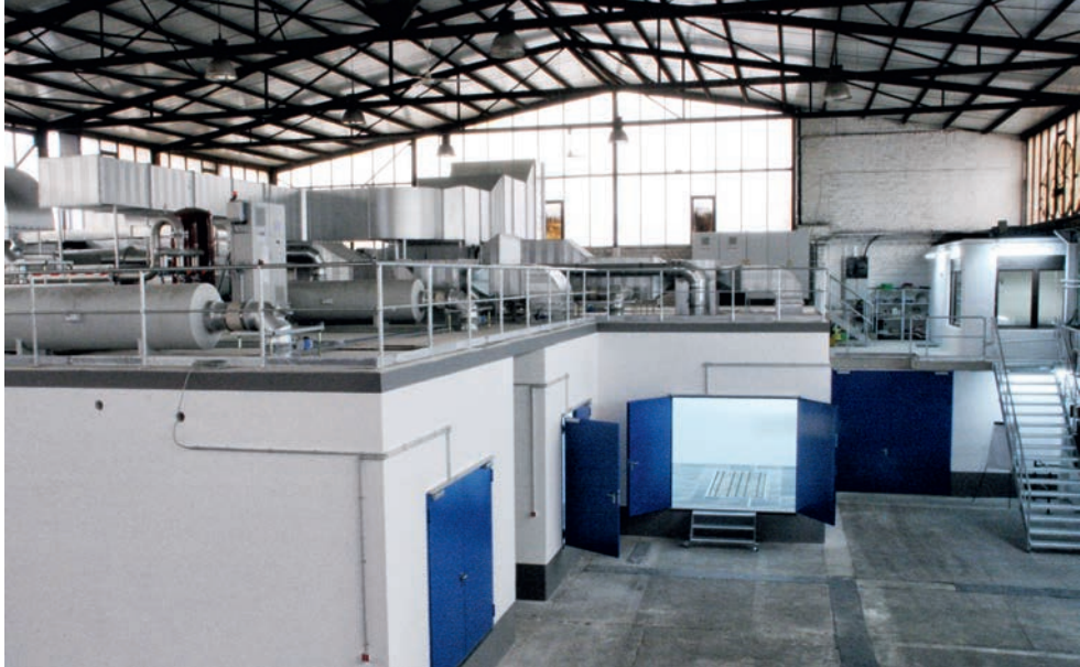
▲ Impressive: Test bay of GVH with three test stands and the power supply equipment (ventilation, cooling, exhaust gas extraction, fuel supply) on the roof.
