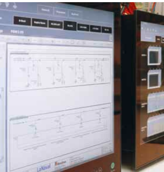
▲ Extremely helpful function in the HMI: Important system details (such as interactive descriptions of the I/O modules) are stored in the SCADA system. This reduces the time required for commissioning or troubleshooting in the event of a malfunction.
