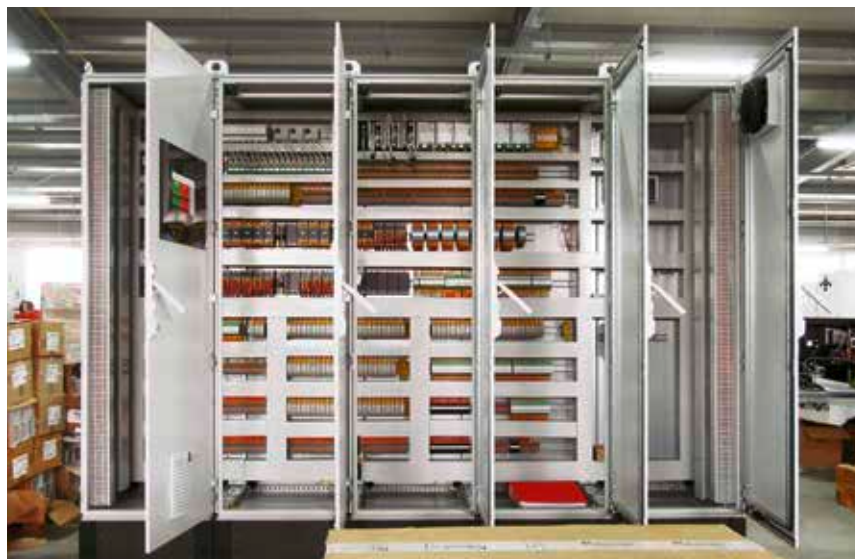
▲ Extensive installation: The control system installation on both special ships consisted of 26 switch cabinets in total. The switch cabinets are assembled in Alewijnse's factory and shipped to the shipyard prewired.
