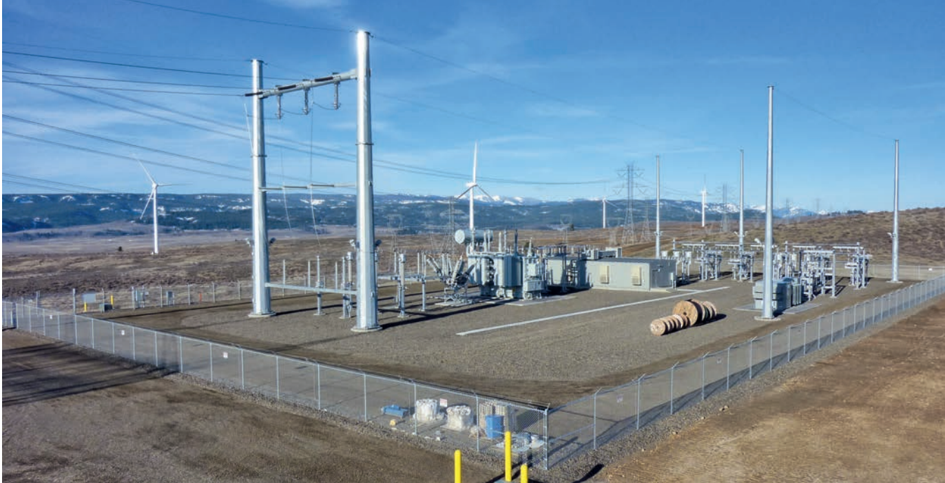
▲ Modules from Bachmann enable grid specific functions with different communication requirements to be provided in just a single system.
